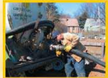
When the holding tank has reached capacity (and the level probe indicates it is full), it can easily be emptied by a roadside tanker, taking only a few minutes.
