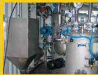
The oxygen-infused stainless steel holding tank periodically mixes and blends the contents. Sizes of the tank can vary to accommodate different quantities of waste production.
